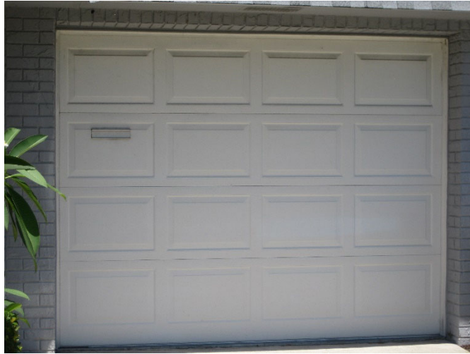
Figure 2 – Typical Garage Door
