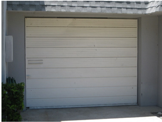
Figure 2 – Typical Garage Door
