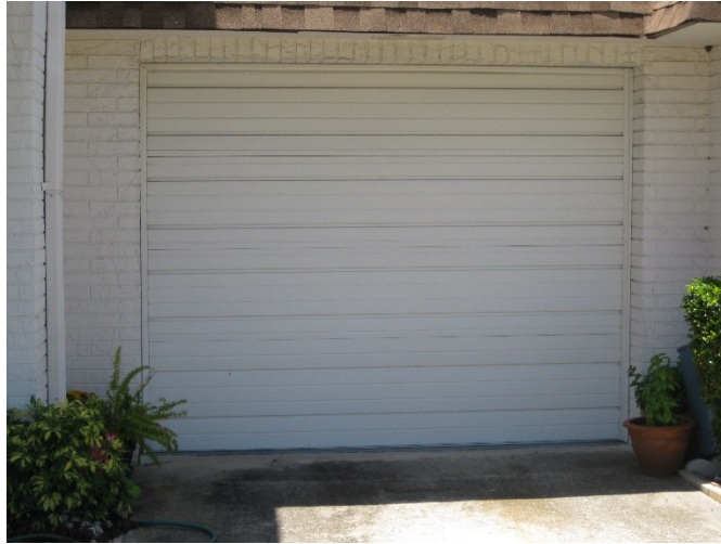
Figure 2 – Typical Garage Door
