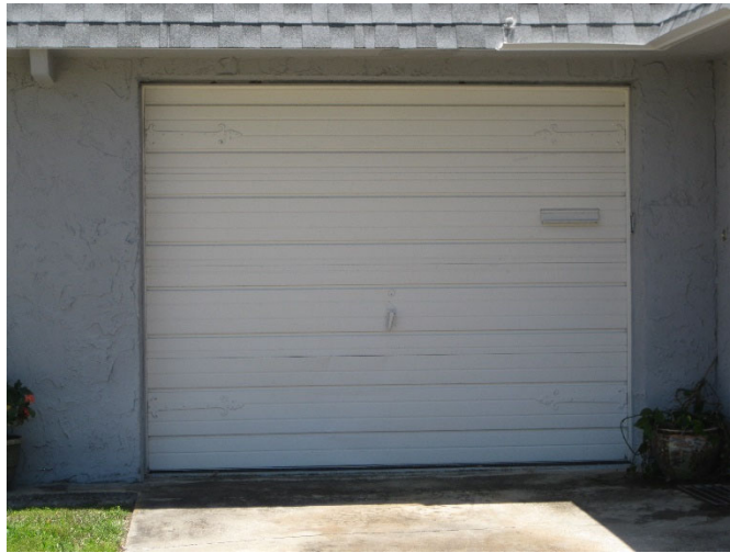
Figure 2 – Typical Garage Door
