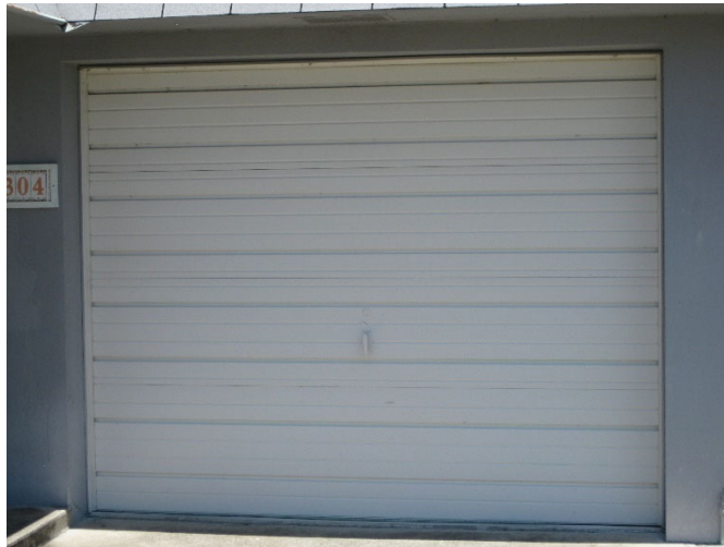
Figure 2 – Typical Garage Door
