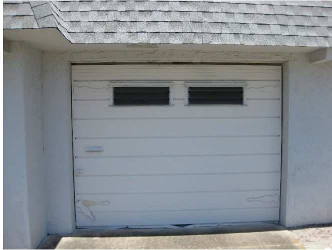
Figure 2 – Typical Garage Door
