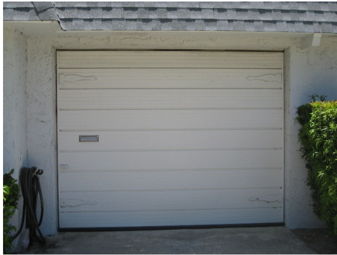
Figure 2 – Typical Garage Door
