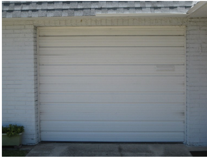
Figure 2 – Typical Garage Door
