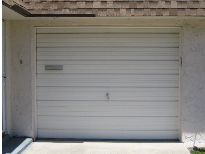
Figure 2 – Typical Garage Door
